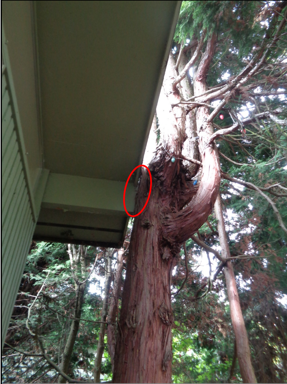
Photo 2: Tree 619, a Hinoki cypress impacting the roof of the house. The red circle indicates the area of contact. This tree was permitted for removal and has been removed.
